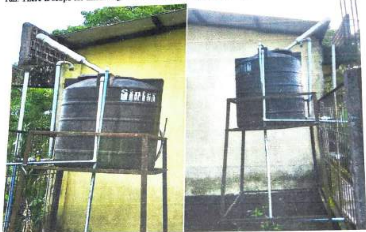
Fig.-5: Rainwater harvesting units
